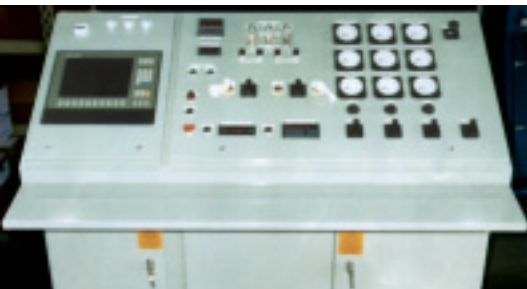
Custom built, electric arc furnace operator's control console
